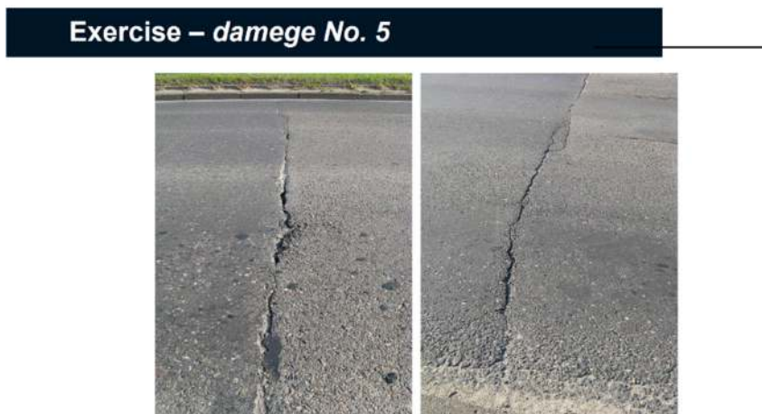
Figure 15 Example of the damage from recognition exercise
